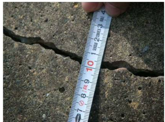
SP275 (L) 柵板ひび割れ
