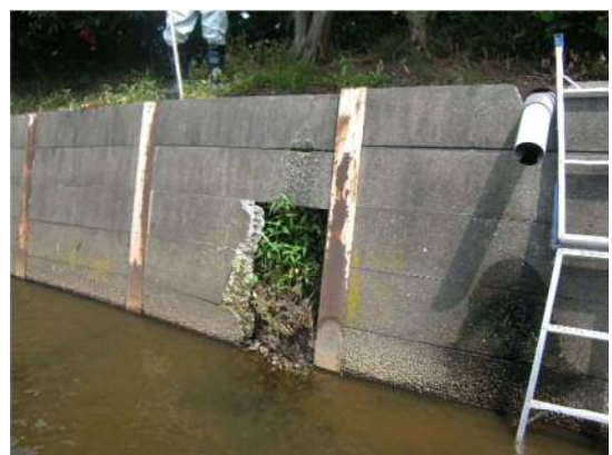
SP694(R) 柵板欠損
